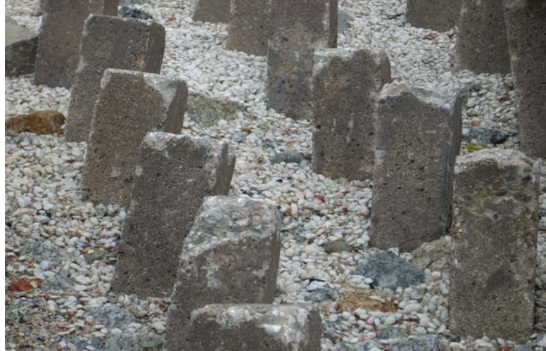
Fig 4. Photograph showing the calcareous deposits on the shore and revetment indicating current erosion and littoral drift
