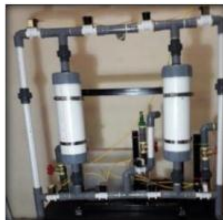
Gambar 9. Unit Iron Removal Filter (IRF)
