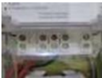
Gambar 15. kWh Meter Keadaan Normal
