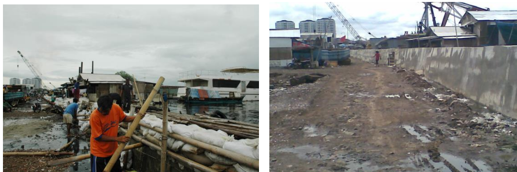
Figure 6. Picture on the left shows temporarily dyke around Pluit area Jakarta using sand bag just after heavy tidal inundation in 2007, while on the right shows one-meter new dyke establish in 2008
