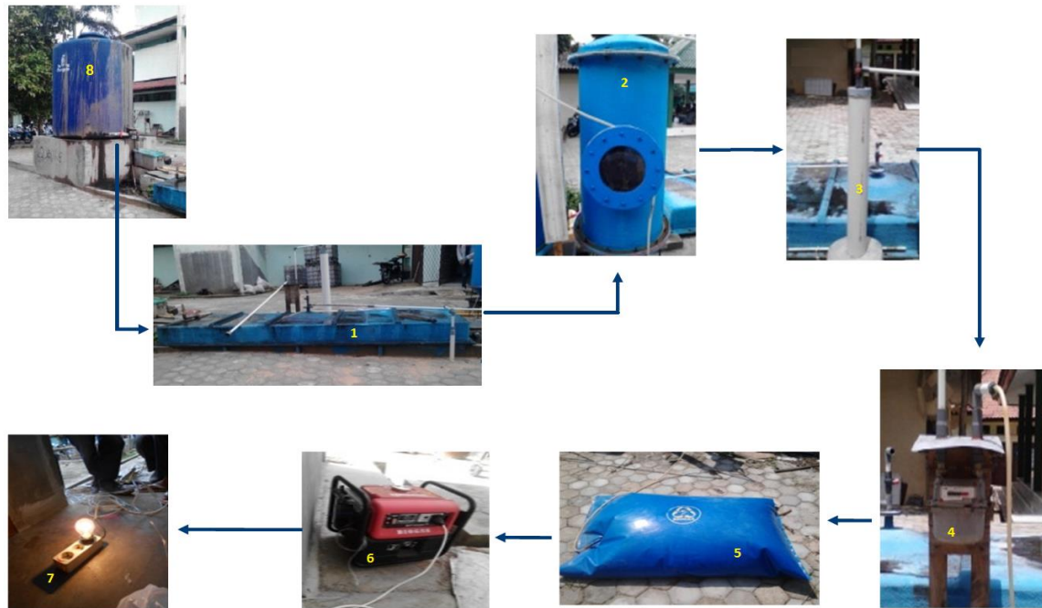
Figure 1. Tools and equipment used in the study, from biogas production to generator testing: 1. Wet anaerobic digester (5 m 3 ); 2. Bio-filter scrubber; 3. Pressure expansion (dryer); 4. Biogas flowmeter; 5. Biogas storage; 6. Generator engine 750-W; 7. Load; 8. Substrate storage tank (5 m 3 ).
