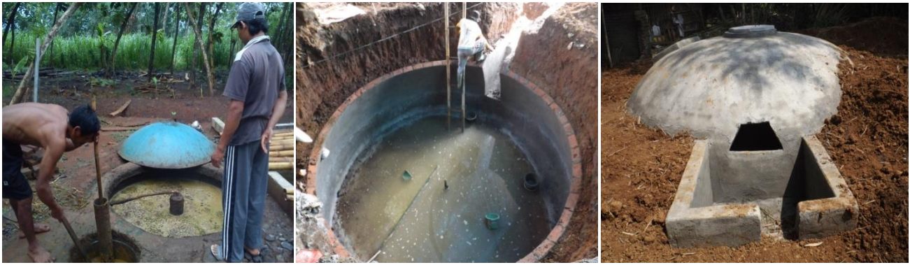
Fig. 3. (a) Fiberglass digester, (b) the construction of a 30 m 3 concrete-fixed dome digester, (c) a finished 30 m 3 concrete-fixed dome digester
