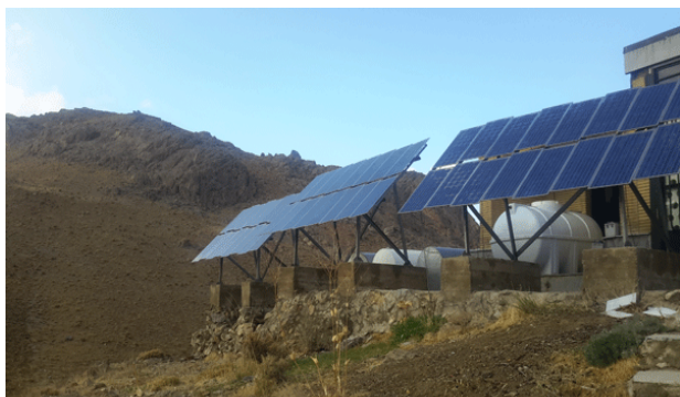
Fig. 7 Electricity to environmental stations.
