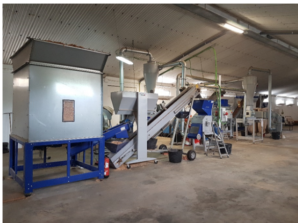
Fig. 1 Biomass prototype plant, production capacity 800 ton of wood pellet/year.
