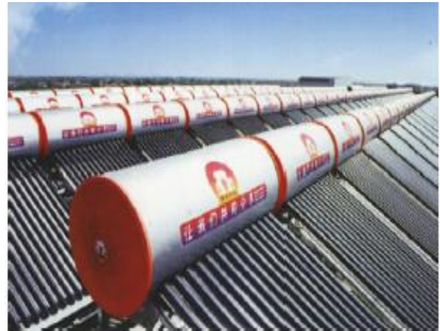
Fig. 7 SWH system installed on a rooftop [26]
