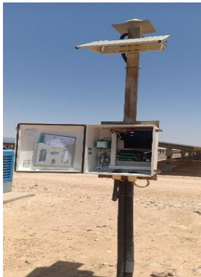
Fig. 1 The Midi Data Logger of the Solar PV Panel System.
