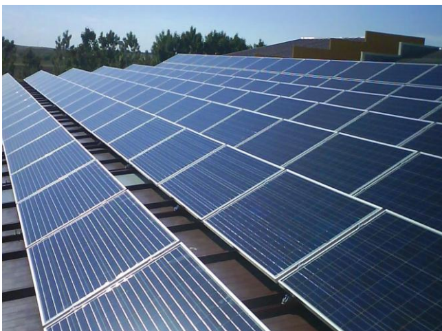
Fig. 6 250 kWp solar plant at Jari hill (Kigali city)
