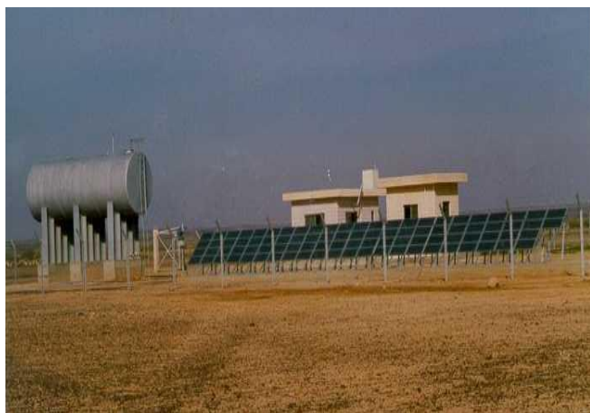
Fig. 1 Sample picture of a typical PV powered water pumping station
