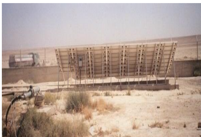
Fig. 2 Sample picture of a typical PV powered water pumping station showing system components
