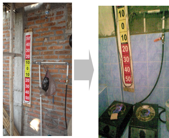
Figure 4. A household put the gas pipeline and manometer at outdoor kitchen in their first five months use of biogas (photo taken in June 2011). (Right). The same household has set ceramics flooring and walling for the kitchen and install two biogas cook stoves for cooking (photo taken in July 2012).
