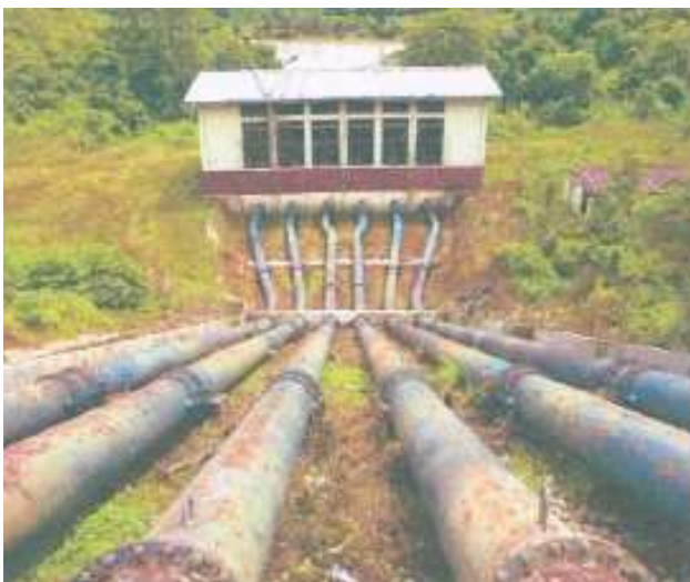
Figure 2. The house of 6 units pumps
