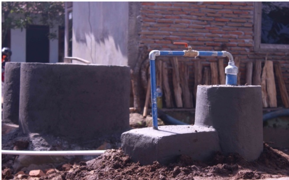
Figure 2. (a) Biodigester Unit
