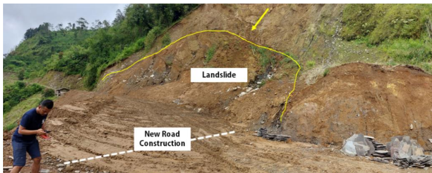
Figure 10. Photo of the Landslide Location at the New Road Construction
