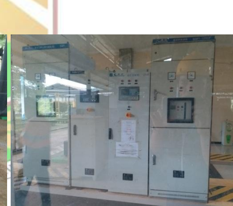
(g) Panel control
