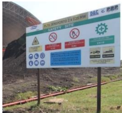
Figure 1. Safety Sign with Physical Work Risk Factors (Source: Personal Documentation)
