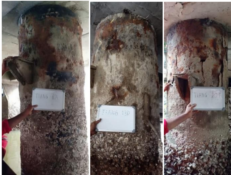
Figure 6. Visual Inspection of Relatively Healthy Jetty Pile (from left to right: 6C, 13D, 20F)
