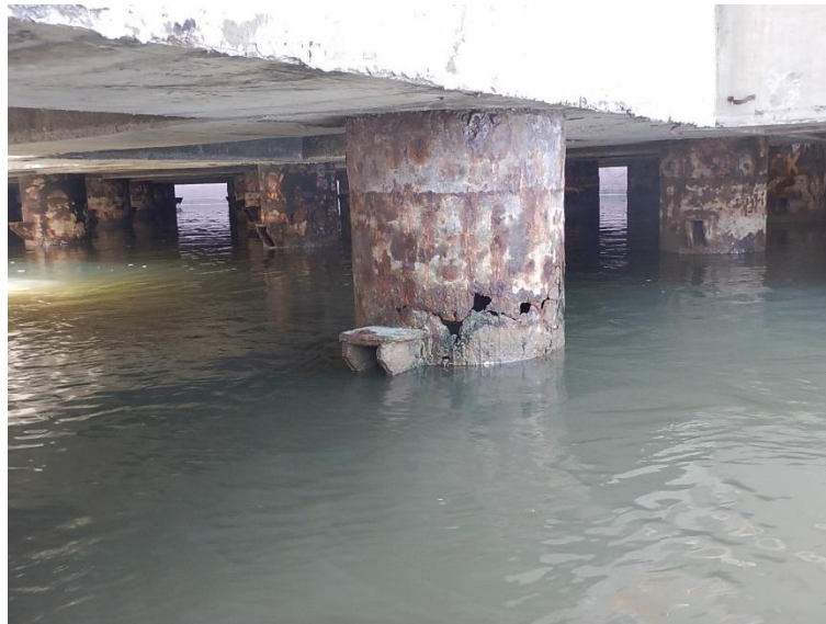
Figure 1. Aged Steel Pile Jetty in Severe Corrosion
