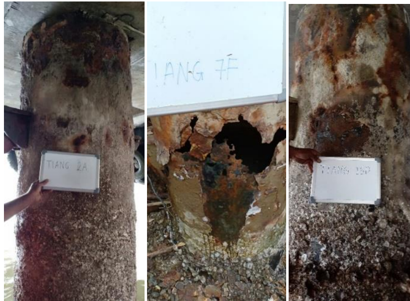
Figure 8. Visual inspection of heavily corroded jetty piles (from left to right: 2A, 7F, dan 15D)
