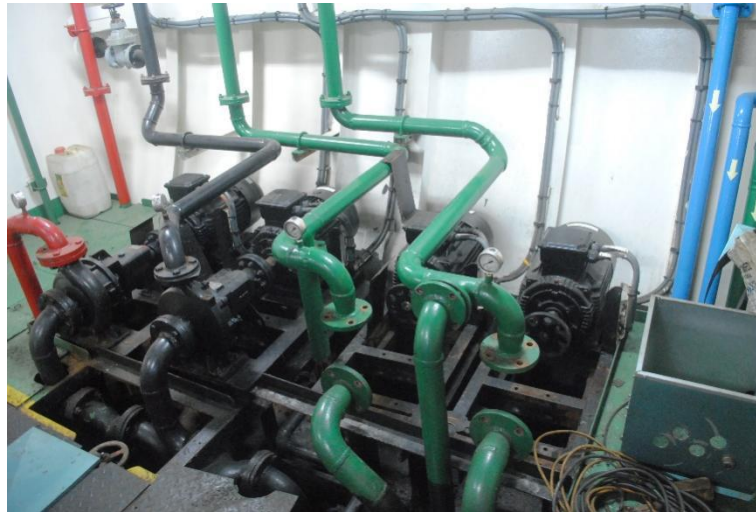
Figure 2. Pumps in the pump room
