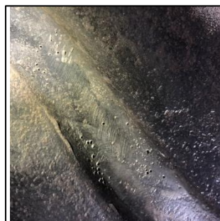
Figure 7. Low Bead Defect
