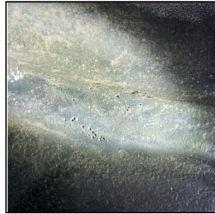
Figure 5. Surface Porosity Defect
