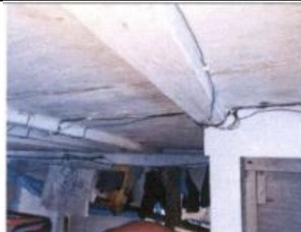
Installation that does not comply with standards
