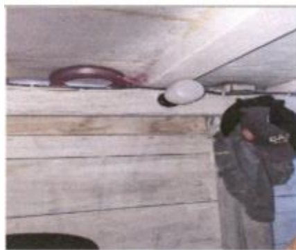
Installation of lights that do not meet standards/attached to flammable wood
