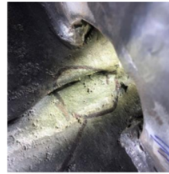
Figure 8. Low Bead Defect
