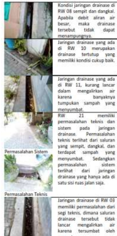
Figure 3. Kondisi drainase streetscape (Rissa & Syarifudin, 2015)
