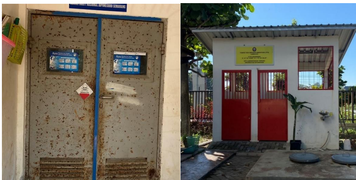
Figure 1. Transfer station of hazardous waste in RSND and UPT
