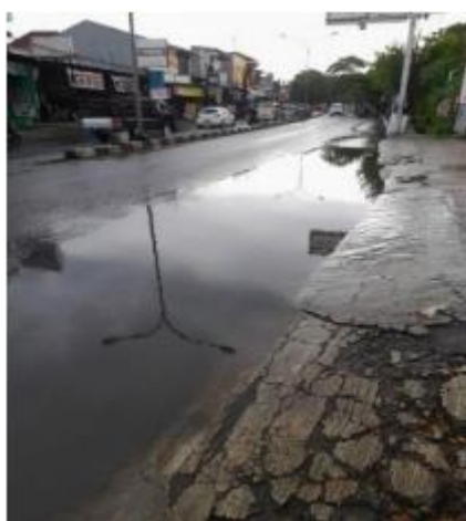
Figure 1. Puddle and flood points on kedungmundu road
