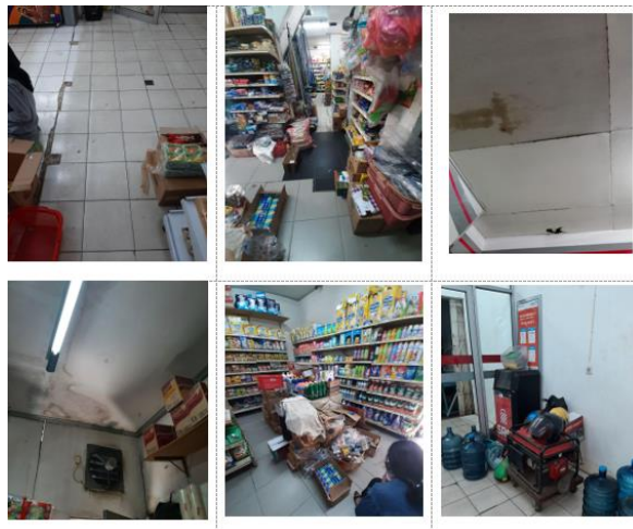
Figure 3. Minor findings on infrastructure and buildings
