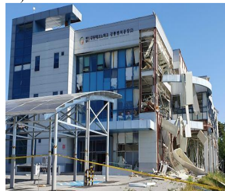
(c) Far-field facade damage observed at approximately 100 m
