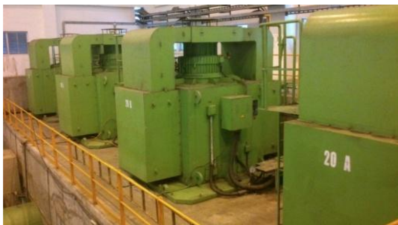
Gambar 2. Circulating Water Pump
