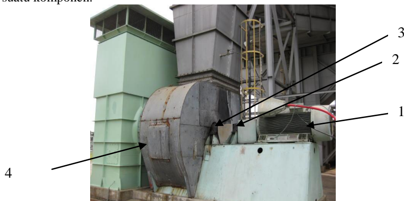
Gambar 1. Blower 22K-102 Force Draft Fan.
