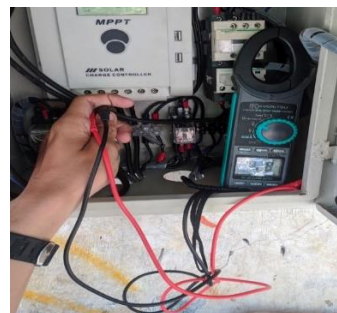
Gambar 3. Pengukuran tegangan-arus panel surya
