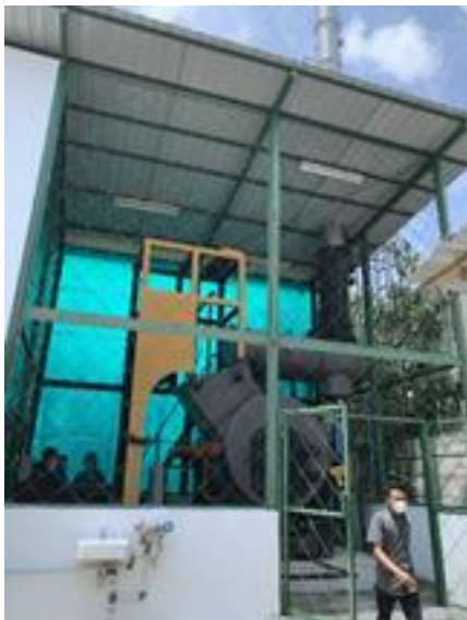
Figure 14. UNS Hospital incinerator tool
